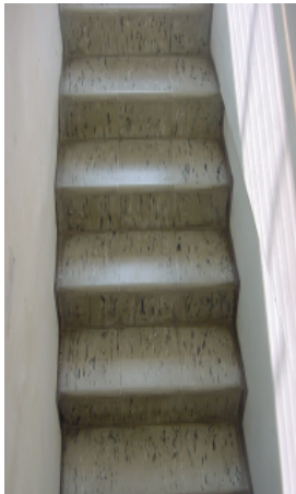
The stairs: slippery when wet!
